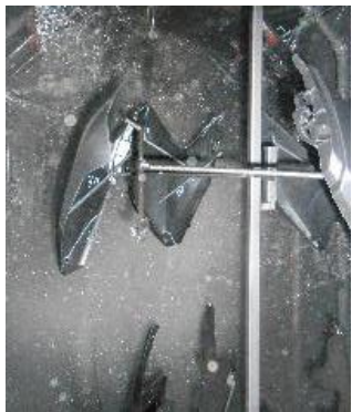
Water Spray Condition
