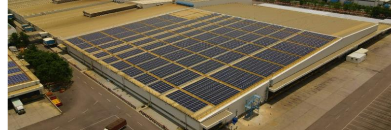
1.6 MW Solar Rooftop on MS Roof
