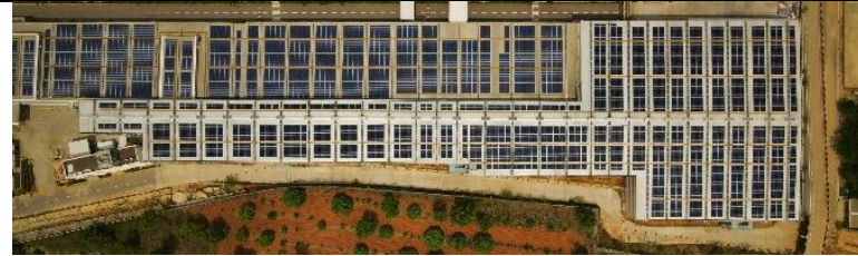
0.9 MW Solar Rooftop on Logistics Warehouse
